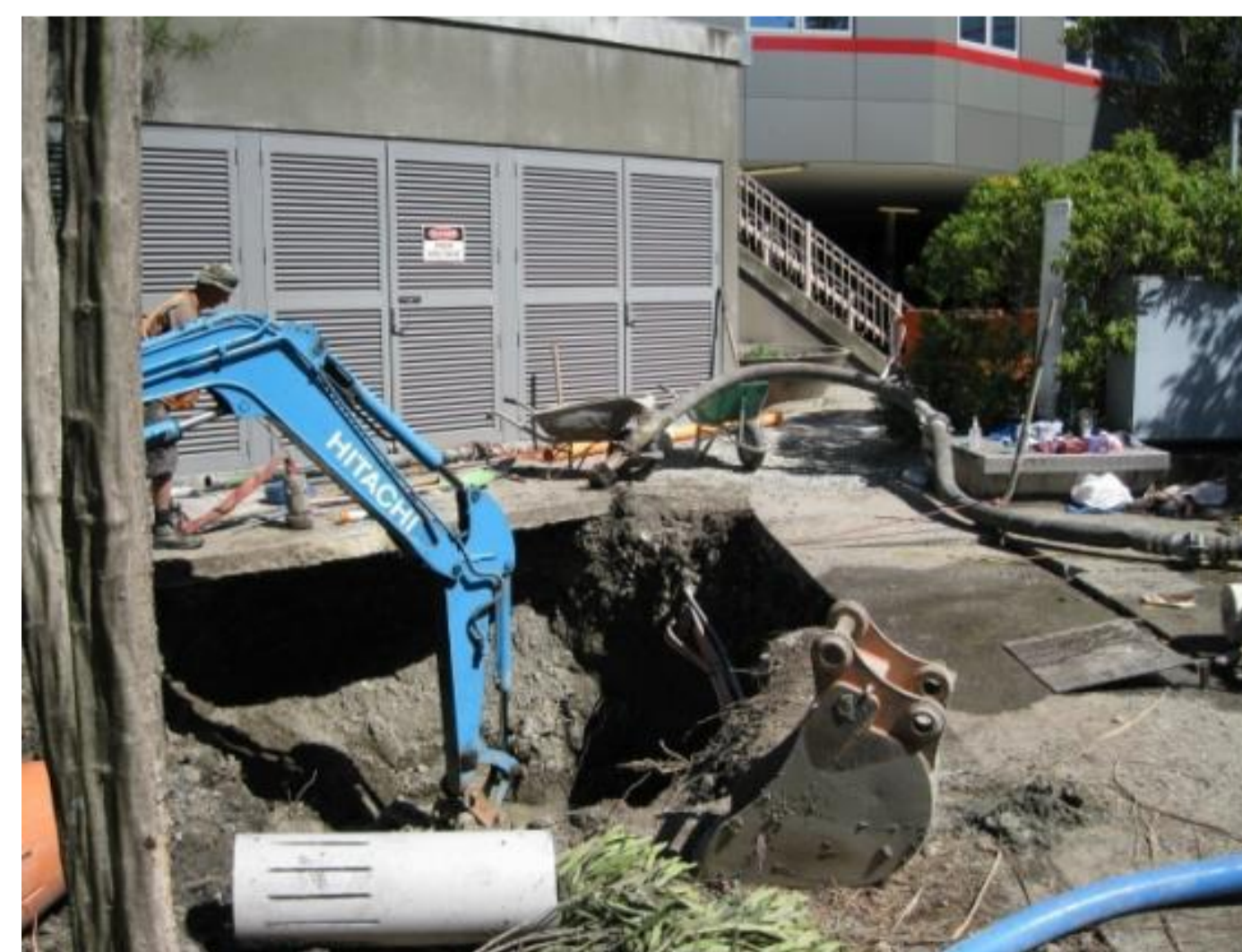
Fig. 2 – Damages to Sewer Lines due to Liquefaction, 2011 Christchurch earthquake [McIntosh, 2012]
